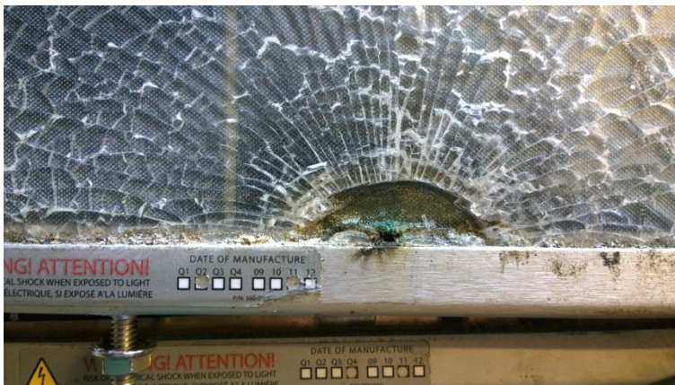
Overheating / Module Failure Example
