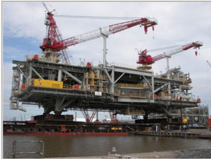
Process module being loaded out at Gulf Island Fabrication. Photo by Jeff Rushing.
