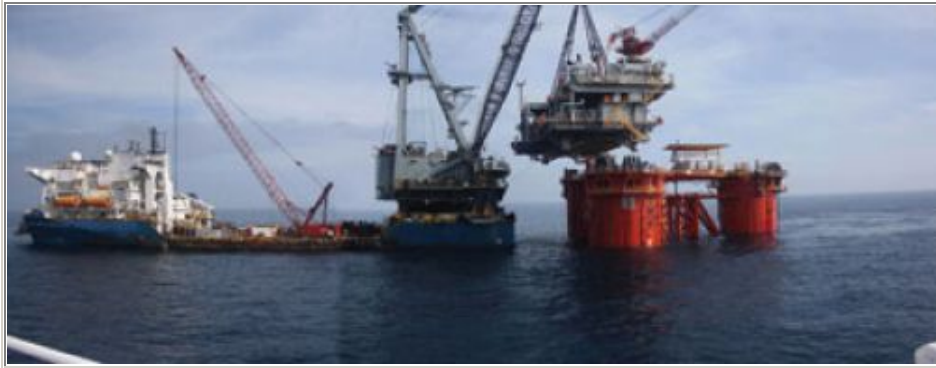
Installation of the process module by J. Ray McDermott's DB50. Photo by Jamie Armstrong.
