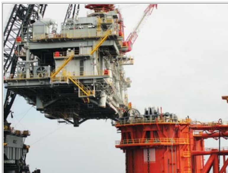
Lowering of the process module on to the hull stabbing guides. Photo by Isidro Rodriguez.
