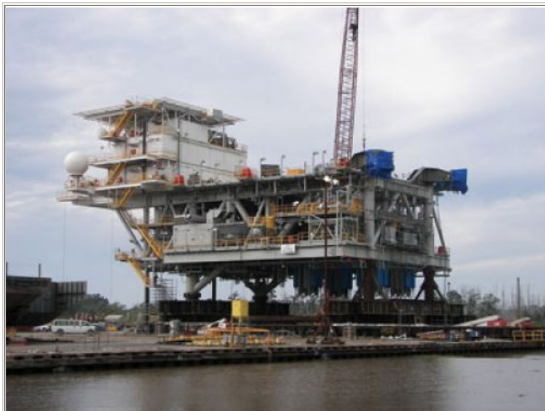
Utility module at Gulf Island Fabrication prior to load out. Photo by Jeff Rushing.
