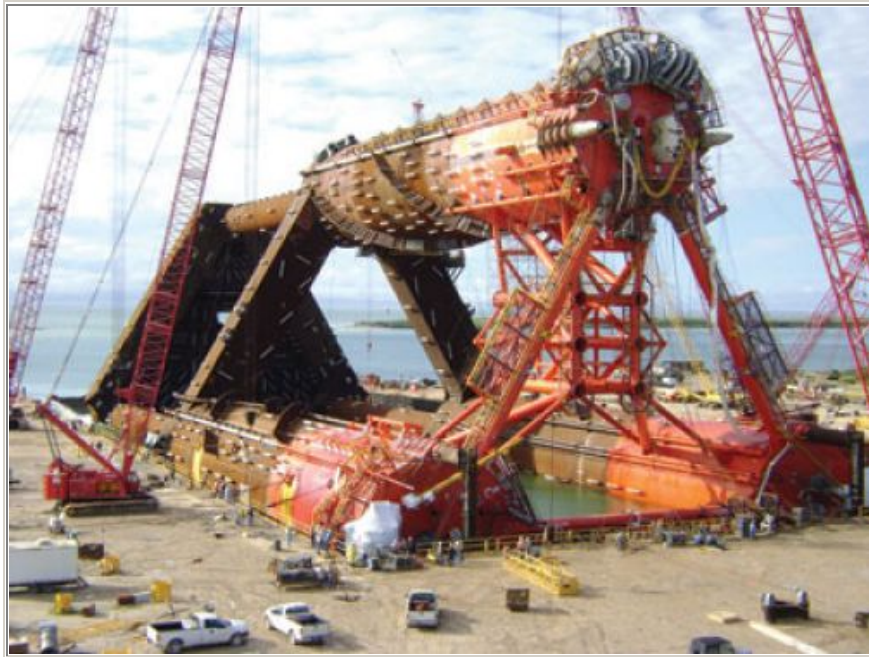
Titan hull floating horizontally in graving dock at Gulf Marine Fabricators prior to sailaway.
